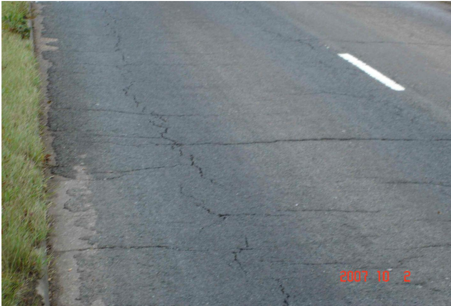
Figure 2.9 Longitudinal and transverse cracking on a minor road
